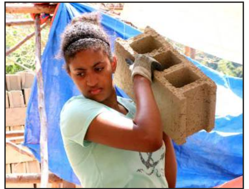
WA sophomore Abigail Lopez passes a cement block on the church construction site. Afternoons were very hot and humid.
