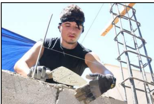
Mickel Arce ('17) helps build a cement block wall on Marcilla church during our 2016 mission project.
