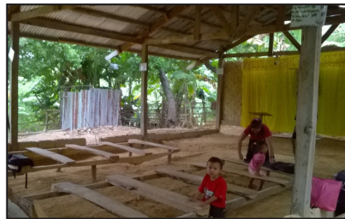
The Marcilla congregation has already torn down this rough structure and begun the foundation for their new church.
