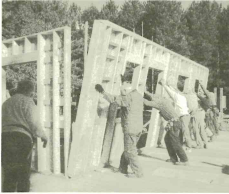
On the second day, volunteers begin tipping up the walls of the Fireside Lodge.
