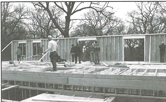
Putting the first wall up, with windows already in place, was a landmark step in construction. One week later. . .
